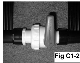
Valve in the closed position Solar heating is ON ( heating )
